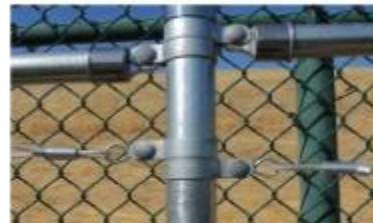
Top rails, tension bands and turnbuckle
