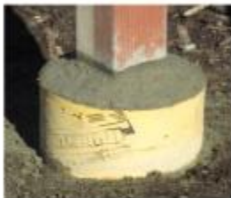
Extend concrete above soil & mulch
